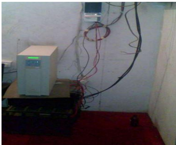
Figure 2: Battery Bank and Converter
